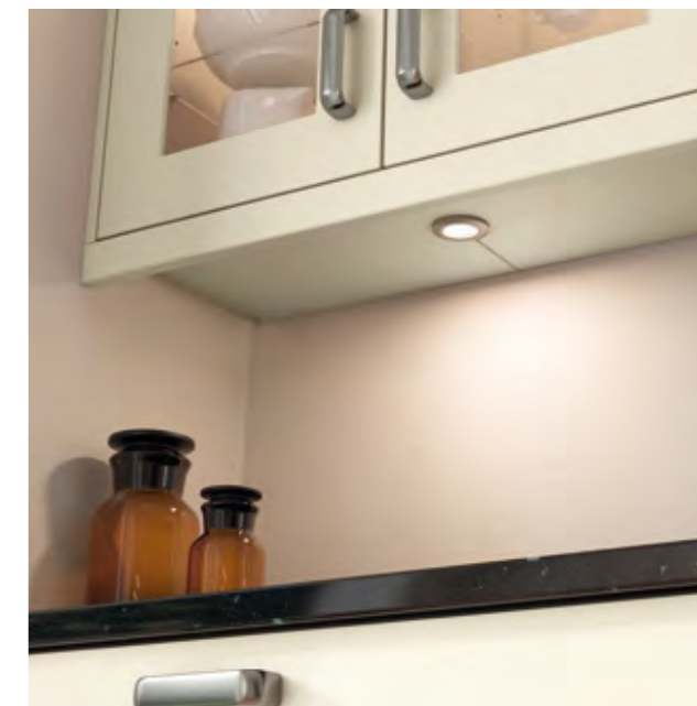
Use downlights under wall units to create additional task lighting, ideal for food preparation in particular.
